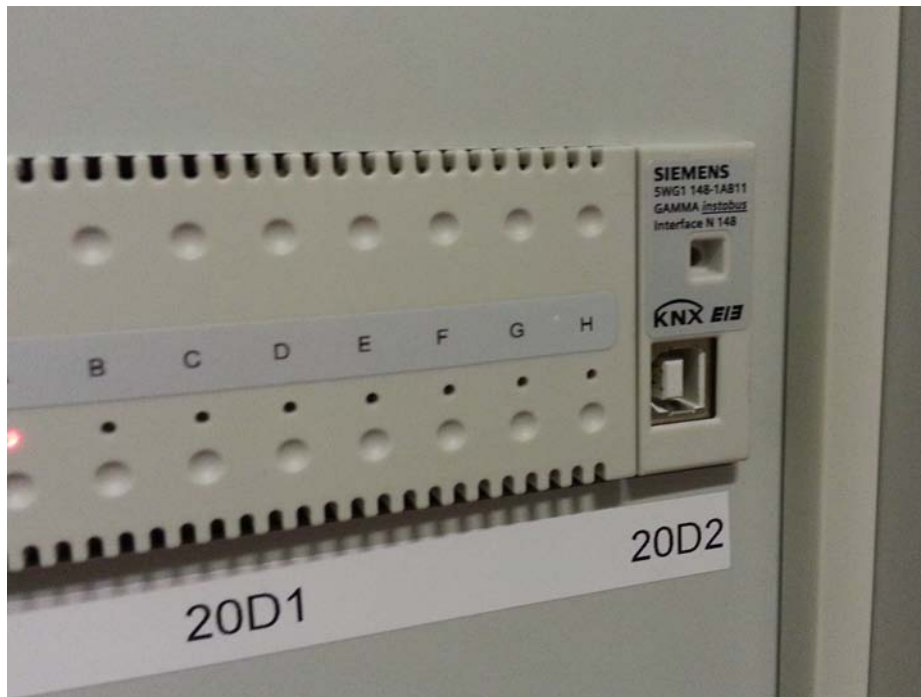
Fig. 12. KNX-USB-gateway installed in a switchboard. Obviously, this gateway was once installed for the ease of initial configuration and later maintenance.
