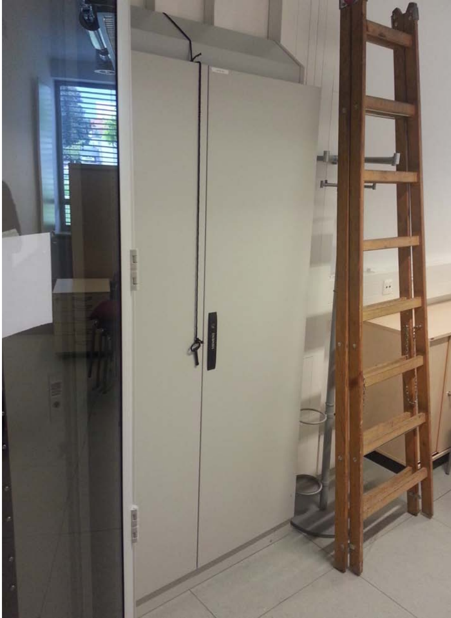
Fig. 13. Electrical cabinet containing the switchboard shown in Figure 12.
