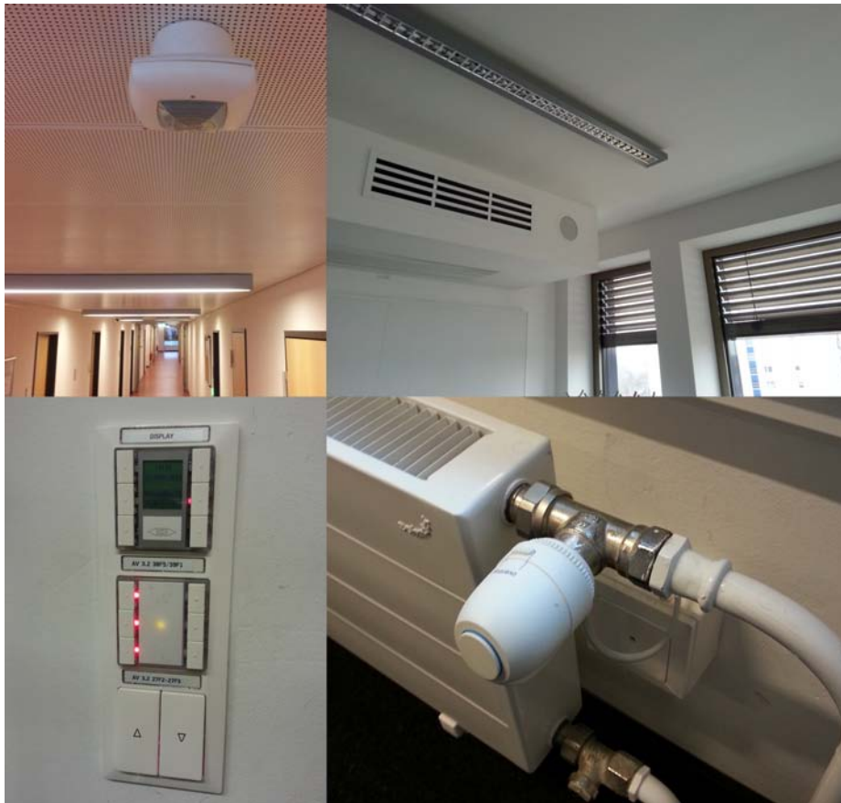
Fig. 8. Visible devices connected by KNX. Top left: Infrared presence detector. Top right: Sun shades, air conditioning and lamps. Bottom left: Control unit for heating / air-conditioning, light and sun shades. Bottom right: heater thermostat.
